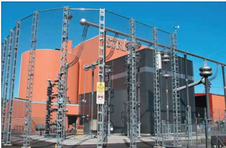
Fig. 1: Illustrating the long-term testing of 800 kV HVDC equipment at the high-voltage test institute STRI in Sweden.
