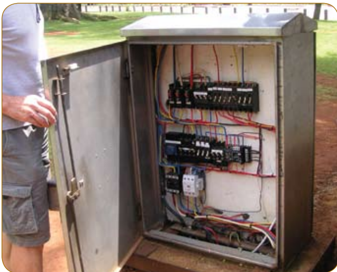
Fig. 2: Examples of safety risks that may be present at public viewing facilities: open and broken electrical boxes and exposed wires.
